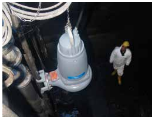
After one year of operation Xylem's Flygt Exporior continues to operate efficiently without clogging.
