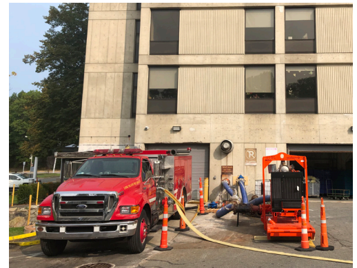
Godwin HL200M 6-inch diesel-driven temporary fire pump providing temporary fire protection at Hebrew SeniorLife.
