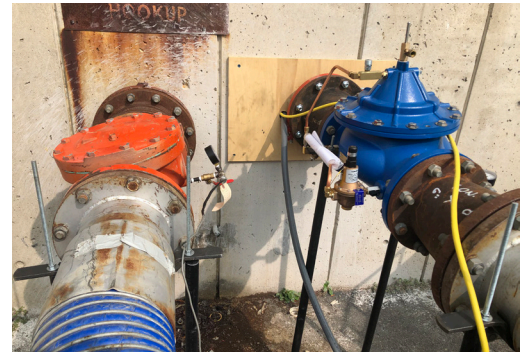
Hospital connection points for the Godwin HL200 6-inch diesel-driven fire pump.
