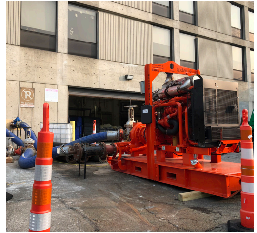
The temporary fire protection system remained in place for four weeks during permanent system upgrades.
