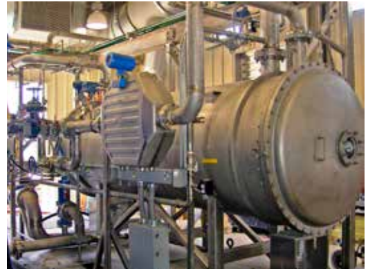
One of the two Wedeco Ozone generators
