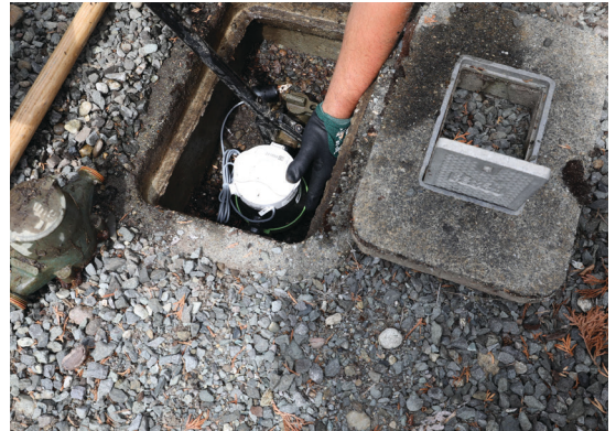
The utility upgrade benefits a growing community with improved reliability, monthly billing, and prompt customer service.
