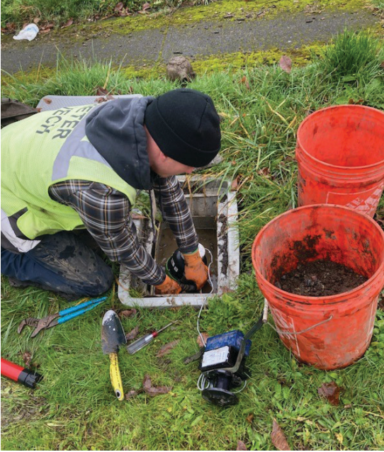
A new advanced meter is installed for reliable two-way communications through FlexNet. The system provides 6.5 million registered reads a day for TPU.
