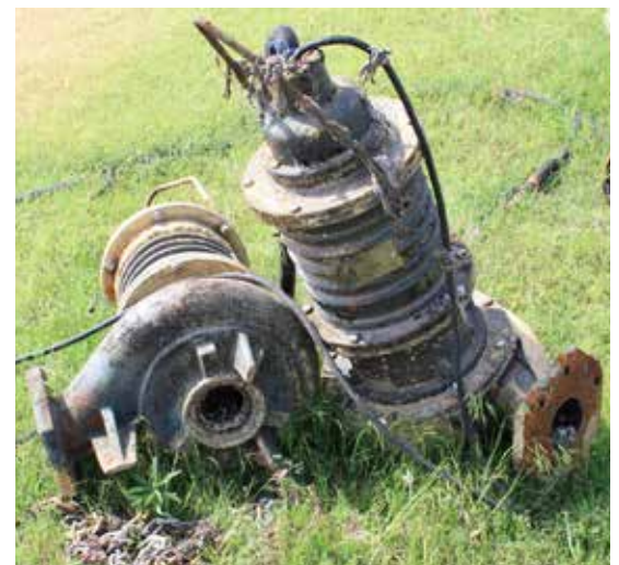
Old pumps with a few rags still hanging on.
