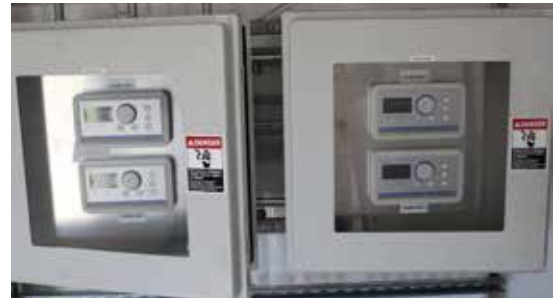
Control panel for each clarifier pump station.
