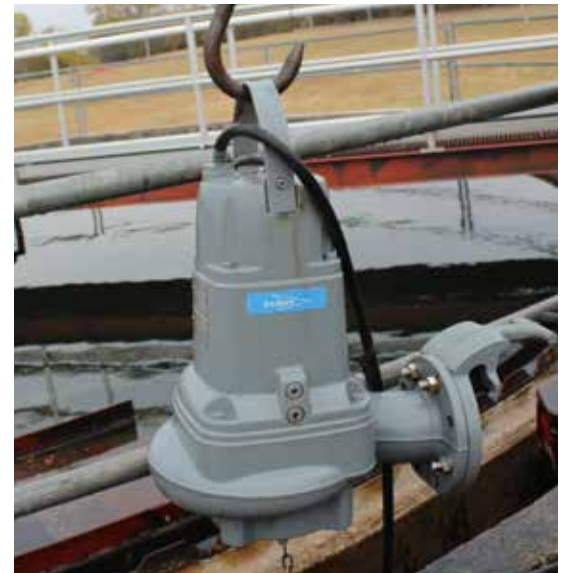
Concertor® pump being removed after 1 month of operation for inspection.
