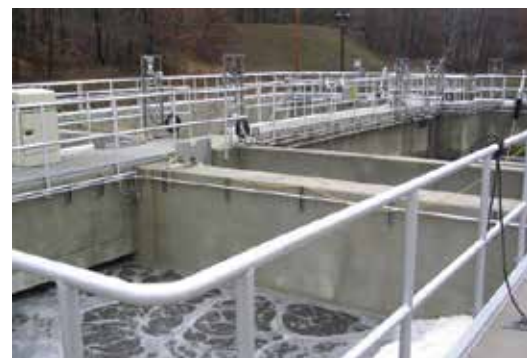
Sanitaire's ICEAS SBR at the St. Joseph Sanitary District No. 1
