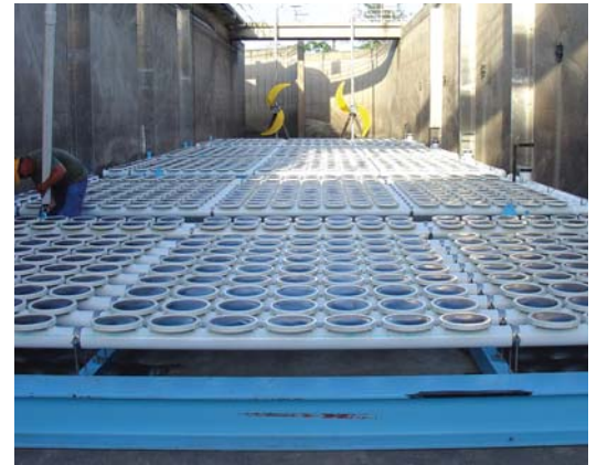
Sanitaire fine-bubble diffusers with removable 9" Membrane Disc Aeration Heads being installed. The two Flygt mixers fitted with banana blades are visible in the background.
