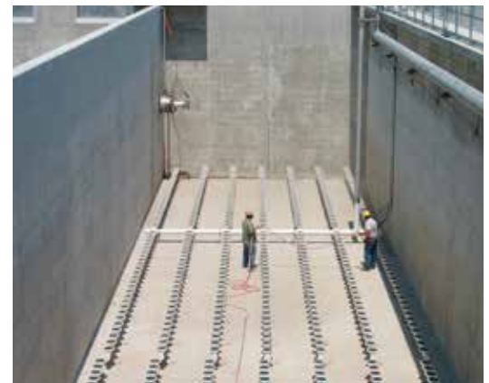
Aeration basin equipped with Sanitaire fine bubble diffusers.
