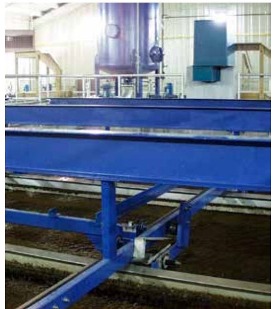
The Leopold Clari-DAF system at work
