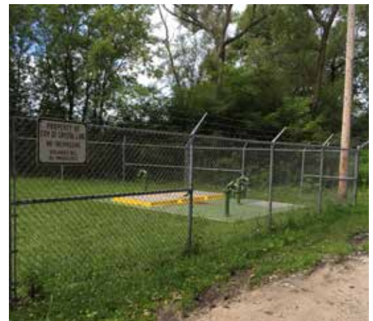
Crystal Lake pump station
