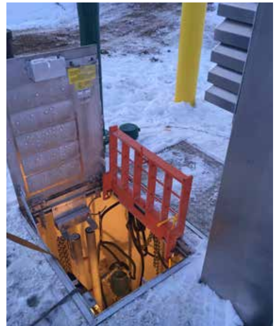
A ground level view of the TOP fiberglass station, which is equipped with Concertor pumps.
