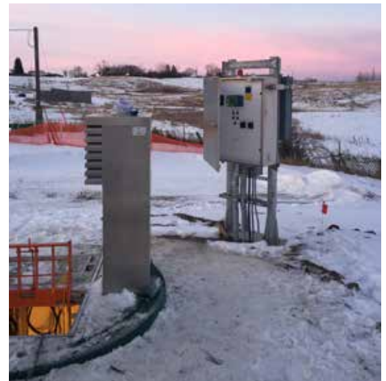
The MultiSmart controller panel is located just outside of the TOP fiberglass station for easy access.
