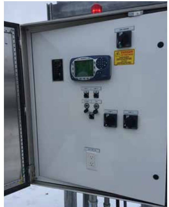
The utility added MultiSmart controllers so staff can more proactively maintain the facility’s assets and optimize energy and performance.
