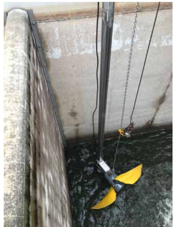
4320 mixer inside the tank
