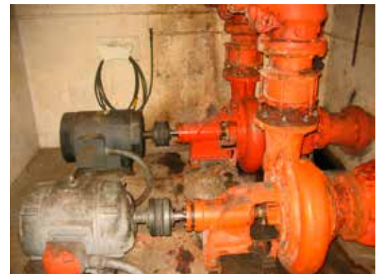
Parts for the original pumps at Ross Street Station were not readily available, causing long lead times for repairs.
