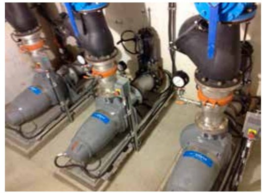
Flygt NZ-3171 pumps installed at Ross Street Station
