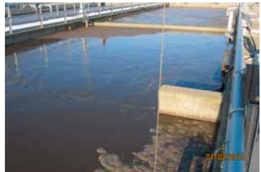
Nine Springs WWTP is an enhanced biological phosphorus removal (EBPR) conventional activated sludge facility. Far Basin: Aeration Basin. Near Basin: Biological Selector Basins. Ripples created by the mixers can be seen on the surface.
