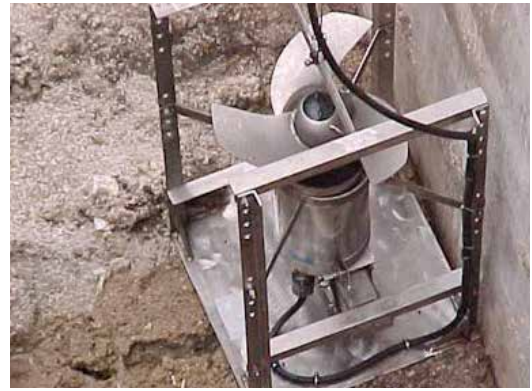
The Xylem Flygt Porta-Cleanse stand mounted Flygt mixer being lowered into the wet pit.
