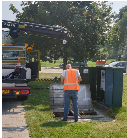
Planned maintenance of a pumping station in Goes, planned and carried out using XDM.
