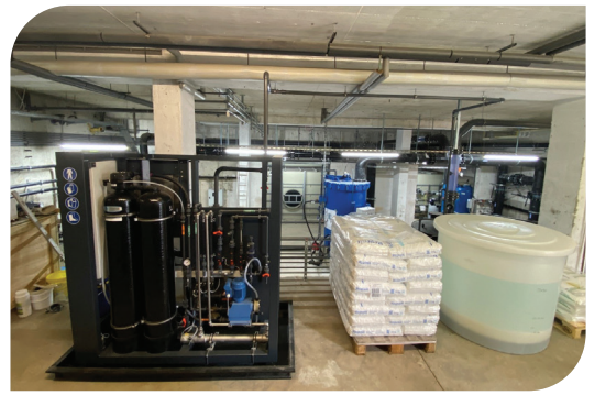
Installed OSEC B-Pak system
