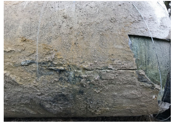
The SoundPrint AFO monitoring platform identified increasing wire break activity on this pipe in early 2020. LHPWSS' decision to replace the pipe prevented a potential catastrophic failure.
