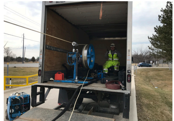
Top: With monitoring data, LHPWSS can conduct selective, proactive repairs rather than replace the entire pipeline.
