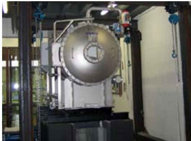
Ozone Generator Type WEDECO PDO 2500
