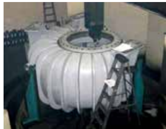
Restoring the fit, flatness and parallelism of the feet and casing faces on the casing and suction nozzle from a 66 x 48 WSYAV pump.
