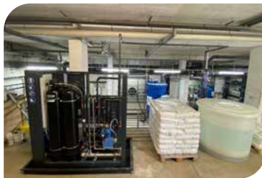
Installed OSEC B-Pak system
