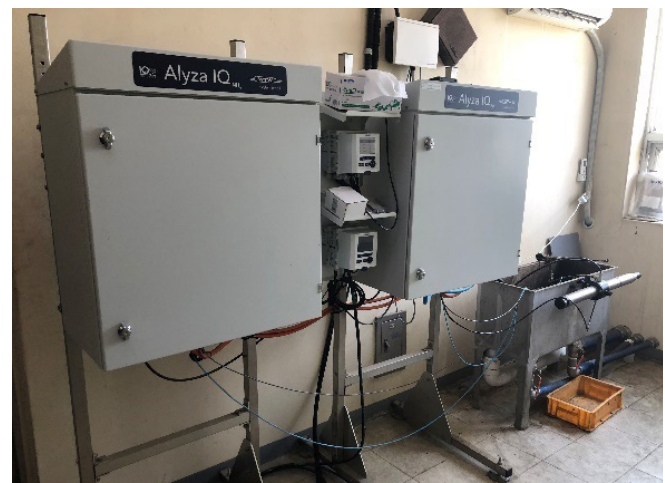
Fig. 6: The WTW Alyza IQ PO4 installed at the Gwangju WWTP
