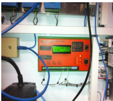
Rain Rate (Inches/Hour) & Rain Total(Inches) was measured and transmitted to the SCADA System
