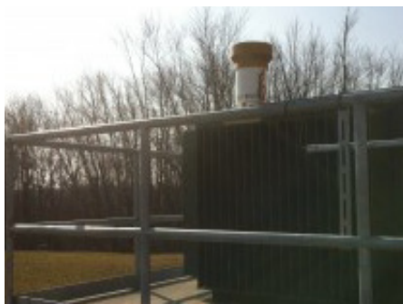
The RG600 Rain Gauge at Des Moines & Mississippi Levee District Pumping Station
