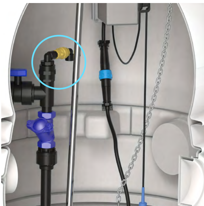
Figure 4.5.1: Siphon breaker located downstream of the check valve.
