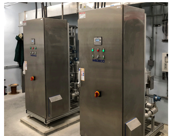
The new water treatment plant incorporates two Xylem Wedeco SMOevo-510 Ozone Generator Systems, significantly improving the quality of the water supply.
