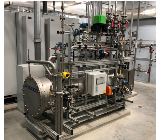
The Long Pond facility treats the water it draws in four separate processes: algae removal, ozonation to improve taste and odor, activated carbon filtration and sodium-hypochlorite disinfection.
