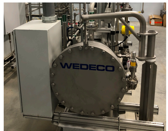
The state-of-the-art Long Pond facility uses the latest control and information technologies so it can be minimally staffed to help keep operating costs and hiring demands down.
