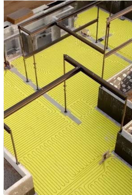
The installation included 5,500 sq. ft. of Rapid Grid under the basement slab and 9,500 sq. ft. of Climate Panels upstairs. PHOTO COURTESY OF NEXTGEN PLUMBING, HEATING & COOLING
