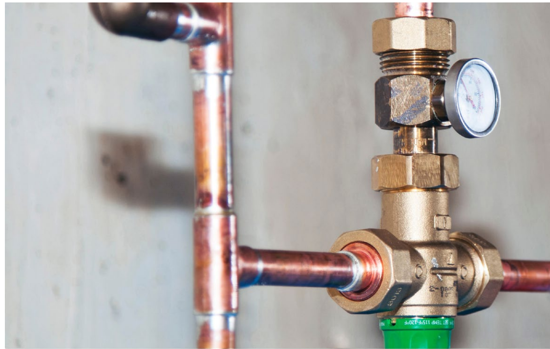
A Taco fixed-temperature mixing valve with temperature gauge is used for a radiant floor application.
