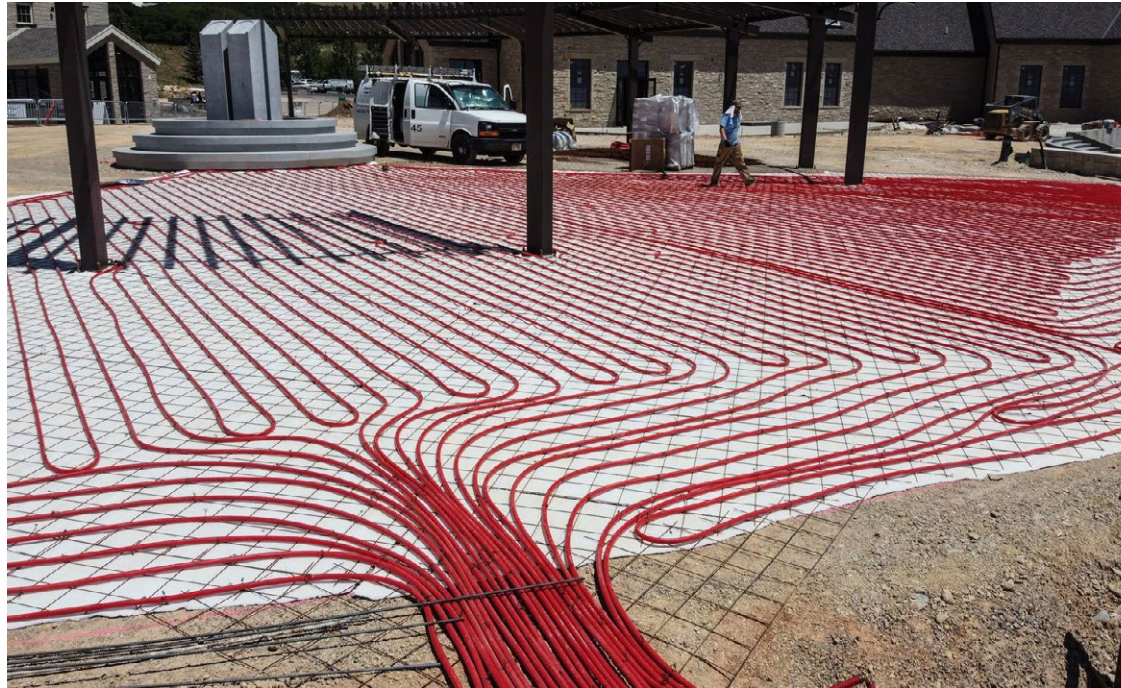
Rehau installed a hydronic snow and ice melting system for This is the Place Heritage Park in Salt Lake City, Utah. Warm water and/or glycol solution is circulated through a network of pipes embedded in the concrete slabs to melt snow and ice above. IMAGE COURTESY OF REHAU.
