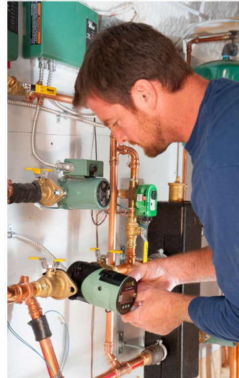
A technician installs a Taco VT2218 delta-T ( \Delta T ) circulator for a radiant heat application. To the right of it is a Taco modulating iValve used to govern temperature for two radiant heat zones.
