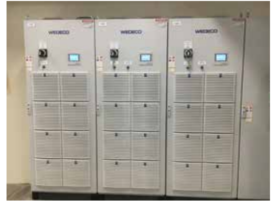
Cabinets house the ballasts to protect important electronics, which are out of the water channel, while also enabling quick access for maintenance.
