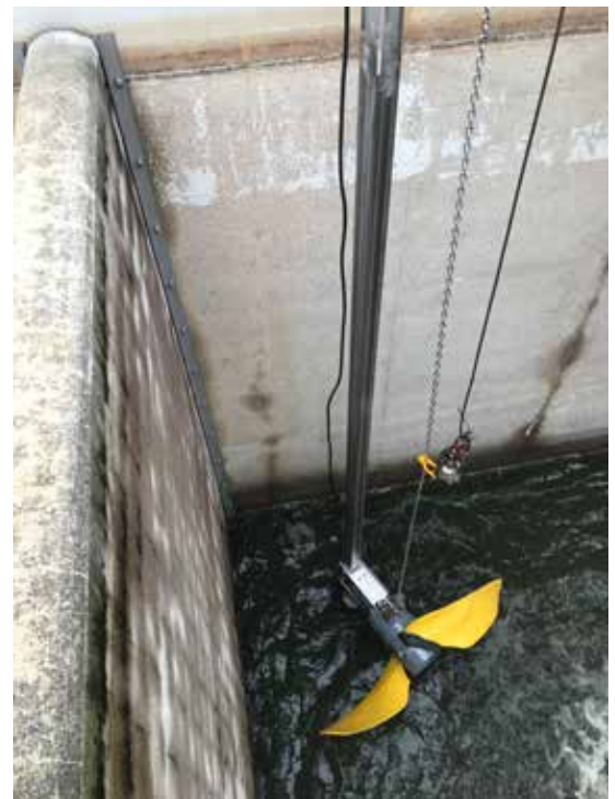
4320 mixer inside the tank
