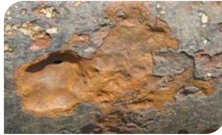
METALLIC PIPE Wall loss
