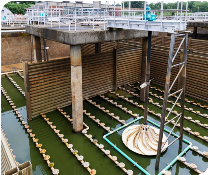
Brockton uses 52 online sensors to optimize aeration control
