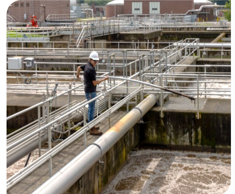
John Downey leads sensor maintenance with best practices to ensure data accuracy and reliability
