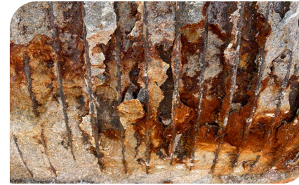
PRESTRESSED CONCRETE PIPE Broken wire wraps
