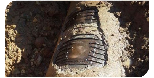
BAR-WRAPPED PIPE Broken bar wraps and cylinder wall loss
